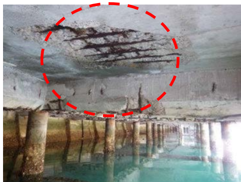
Corrosion of steel bars causes spalling of concrete Example of Port structure
